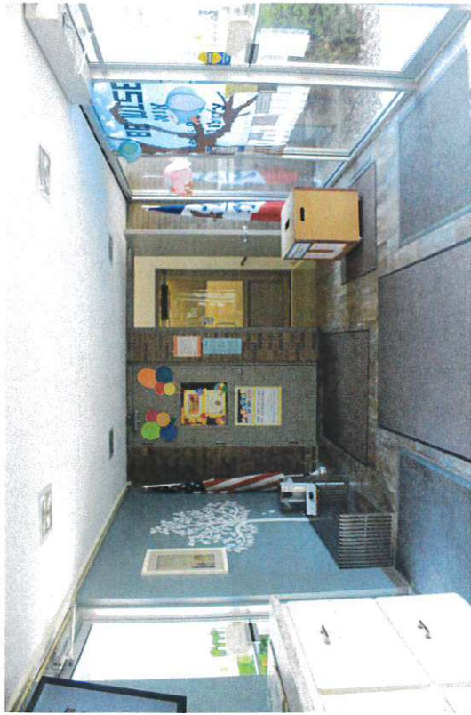
A1 - Entryway Doors to Carnegie Carnegie and Addition sit at different floor heights making circulation throughout the building difficult and not ADA accessible.
