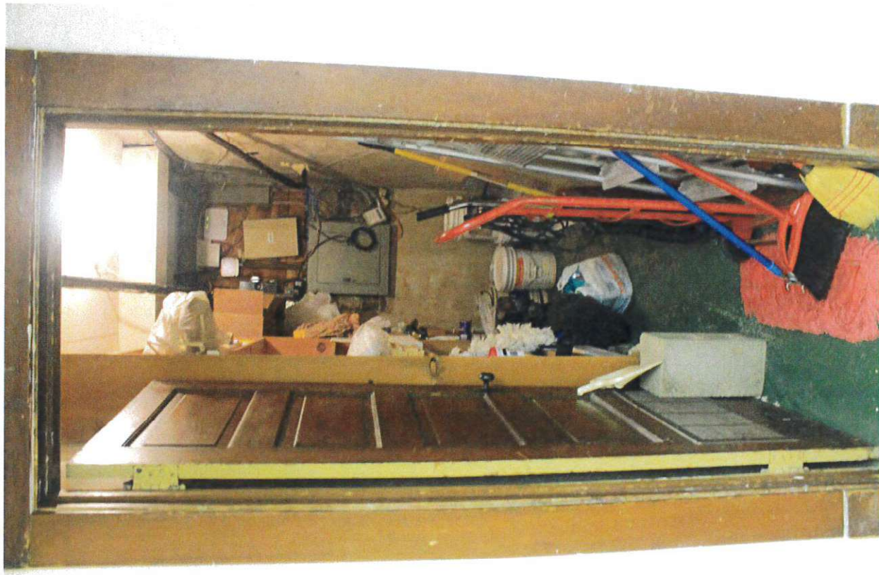
B22 - Janitor's Closet Electrical room is also being used as custodial and IT storage.
