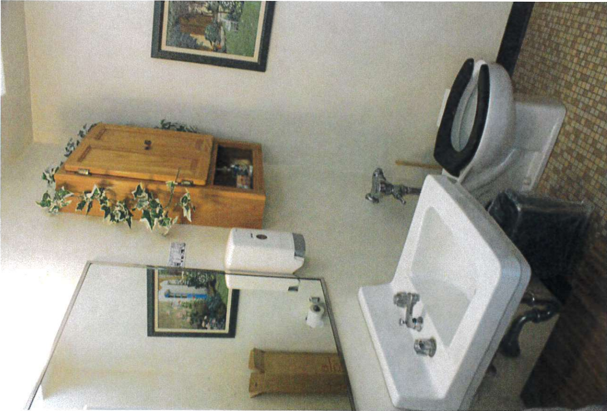
A36 - Addition Staff Restroom Restrooms are not ADA accessible.
