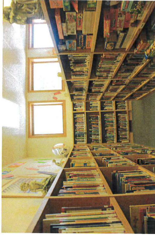
C11 - Book stacks looking South Space between book stacks is not ADA compliant
