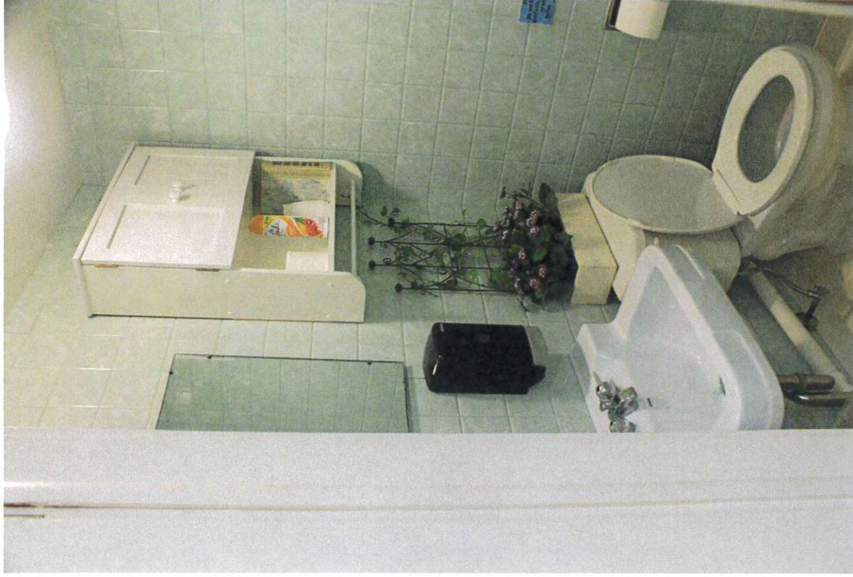
B10 - Basement Restroom Restrooms are not ADA accessible.
